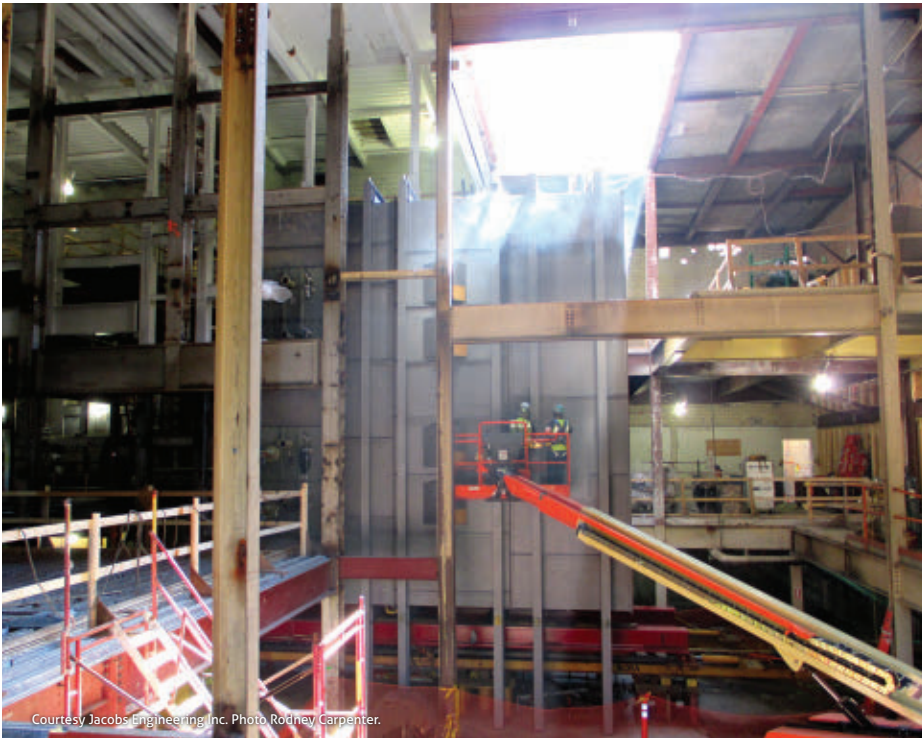
Heat recovery steam generator modules entered Old Main through a roof penetration in September 2015.
